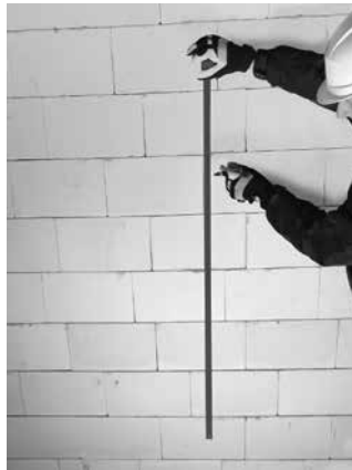
Image 19 Measure and mark out the pipe bracket locations and branch drain tie-ins along the set-out stack path.
